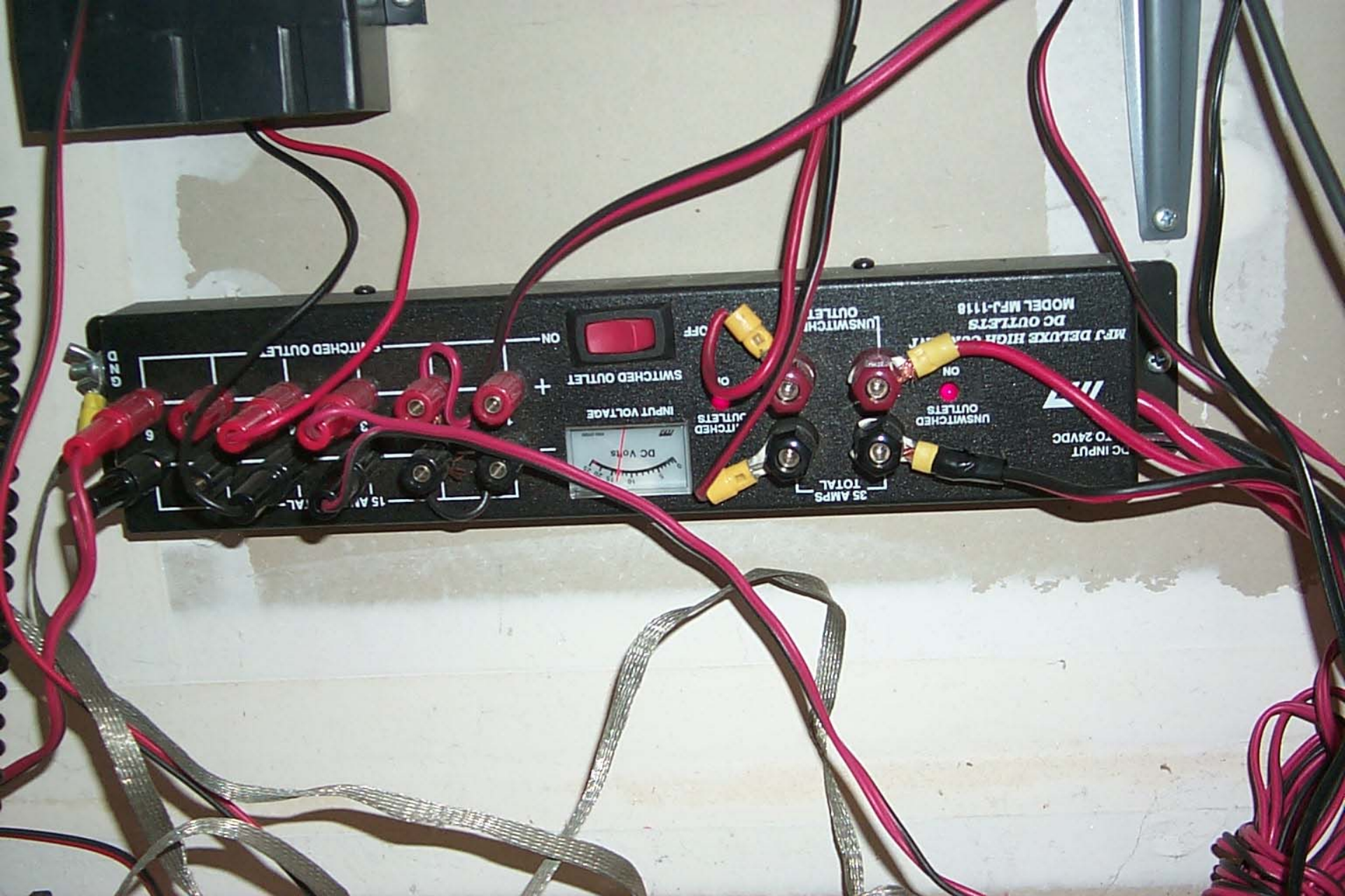
Next is the power distribution panel. The lines on the left are set to handle 15 amps, the right 35 amps.
